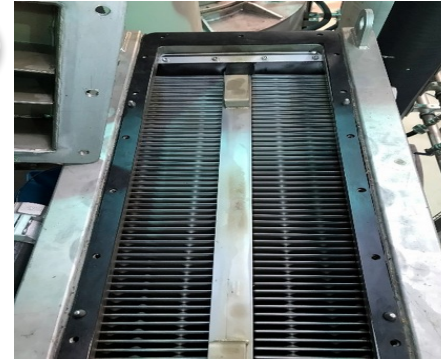
Heat exchanger, 2 years operation, no fouling
